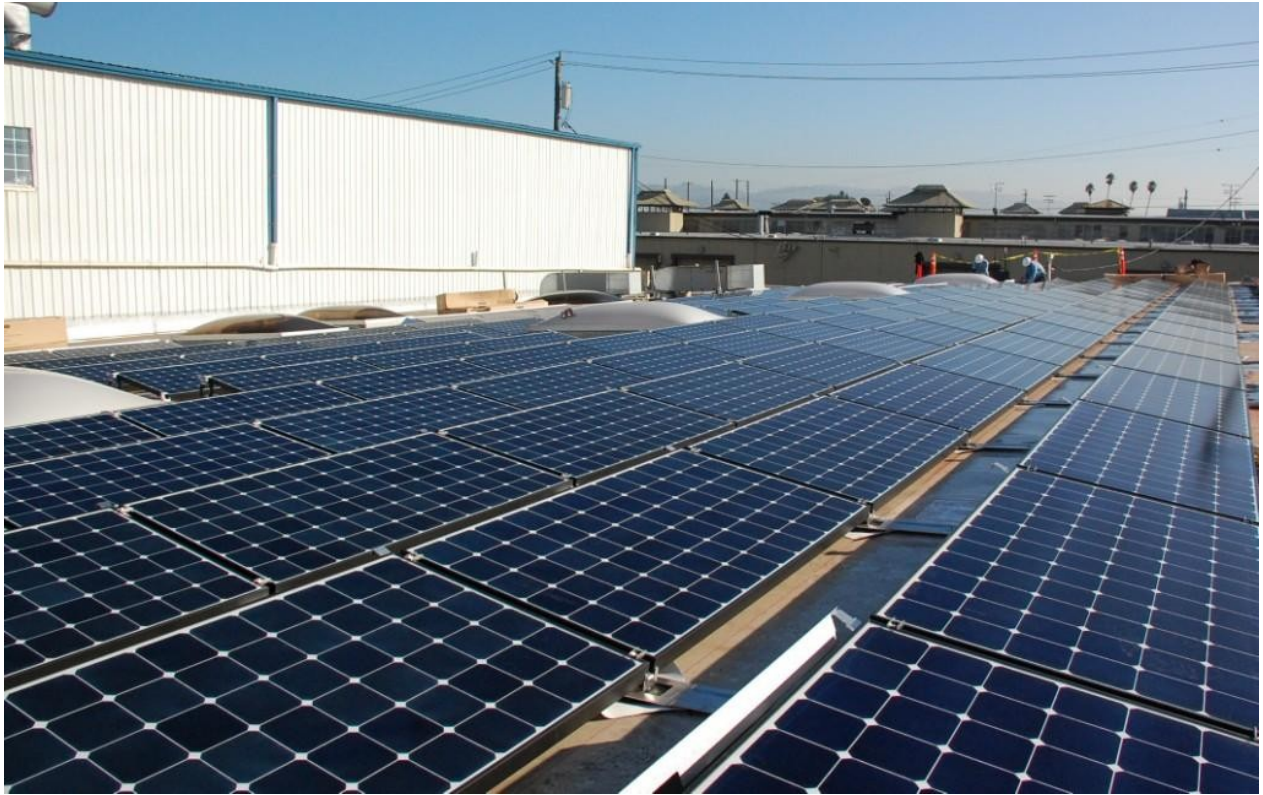
Solar panel array on main roof of Feeney, Inc. facility, Oakland, CA 2011
